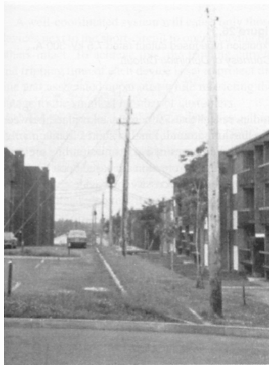
Figure 26.28 MV aerial feeder serving a residential district.
